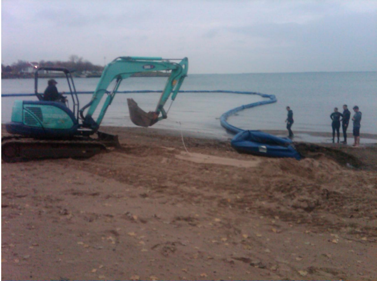
Above: Removal of the barrier in October of 2012. In 2012, Lake Michigan experienced record low water levels. Portions of the barrier were buried by sand due to drifting sand and receding water levels. Heavy equipment was needed to remove the large amounts of sand that accumulated on top of the barrier during the project.
