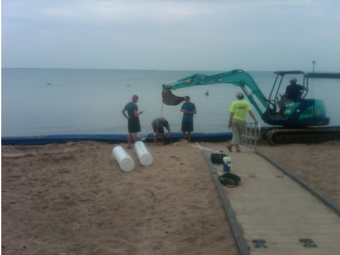
Above: Installation of the barrier in July 2012. Flotation billets are shown in the foreground. The barrier arrived disassembled, and staff assembled the sections on site.
