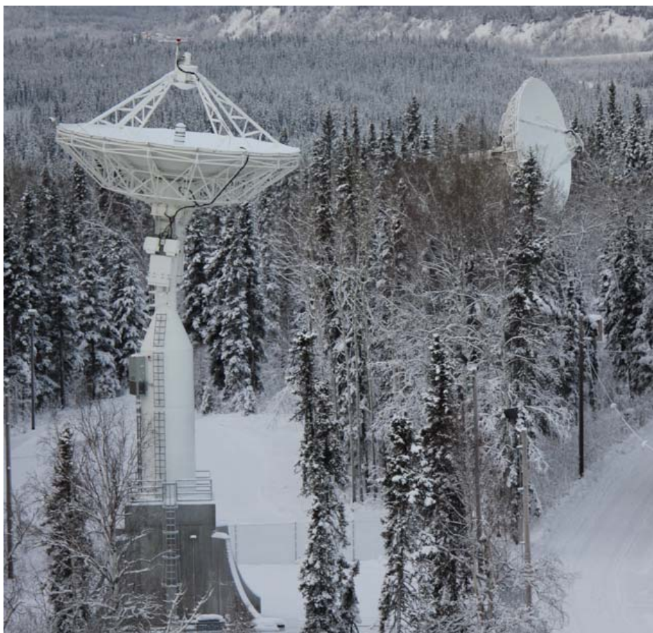
Figure 7-2. New AS3 erected on new foundation at ASF (foreground) Existing AS1 (background)
