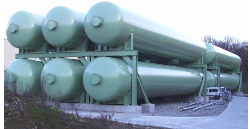
2 MPa gas tanks
