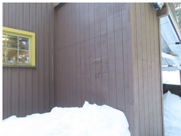
T1-11 Plywood Siding Delaminating
