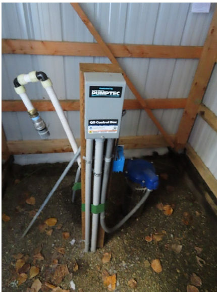
Well Head and Well Pump Control Box
