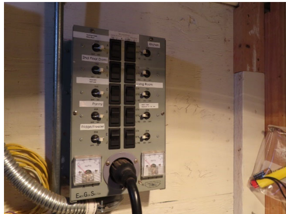
Generator Switch Box
