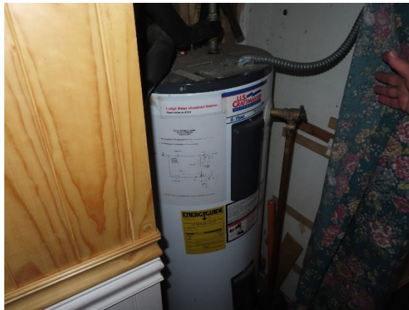
50-Gallon Lower-Level Water Heater Manufactured in 2003
