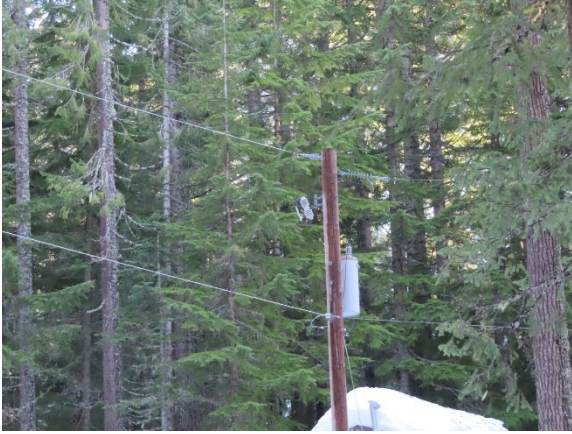
One of Three Pole-Mounted Transformers
