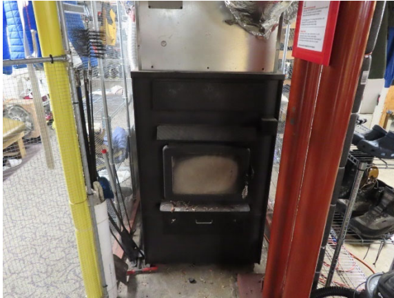
Basement Wood Furnace
