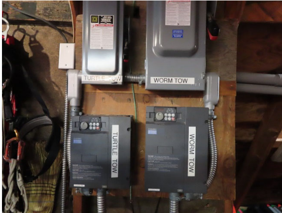
Controls for all 3 Rope Tows
