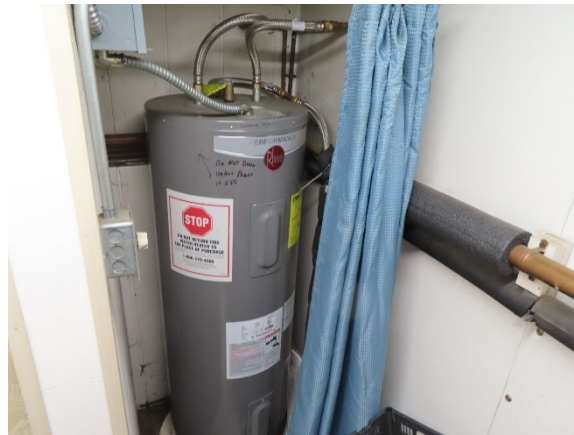
50-Gallon Lower-Level Water Heater Manufactured in 2017
