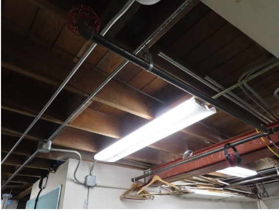
Typical Basement Light
