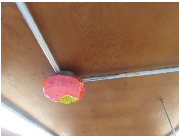
Typical Smoke Detector
