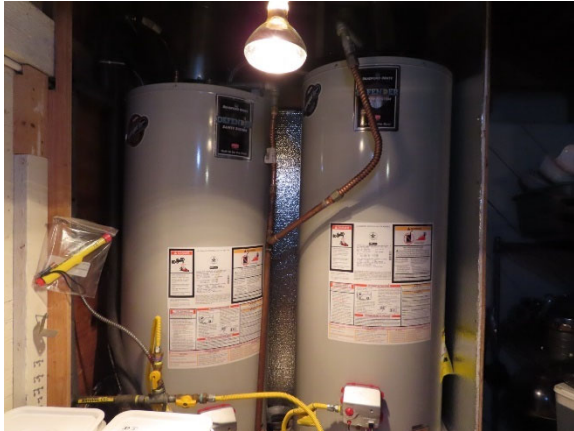
Two Second-Floor 50-Gallon Water Heaters Manufactured in 2018
