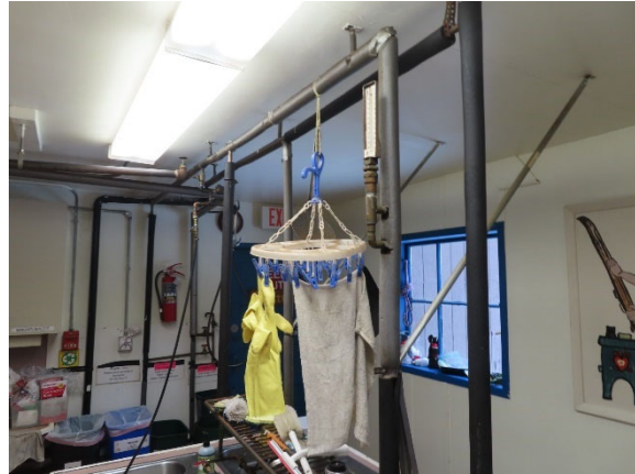
Typical Copper Supply Piping in Kitchen
