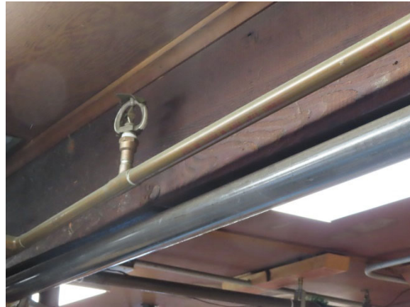
Typical Fire Sprinkler Head
