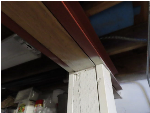
Lower-Level Wood Beam Reinforced with Steel C-Channels
