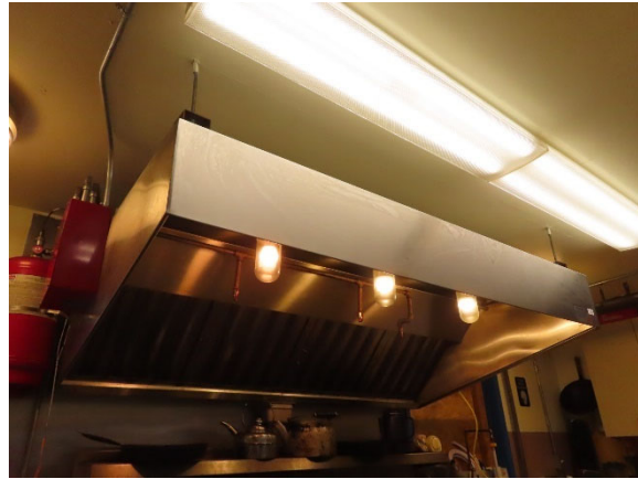
Kitchen Range Hood
