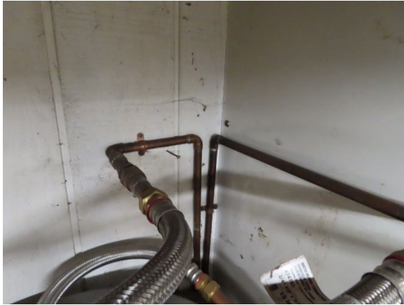
Typical Copper Supply Piping
