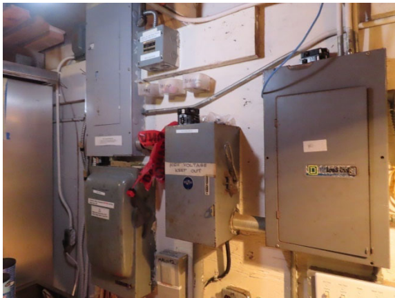
Main Electrical Switchgear and
