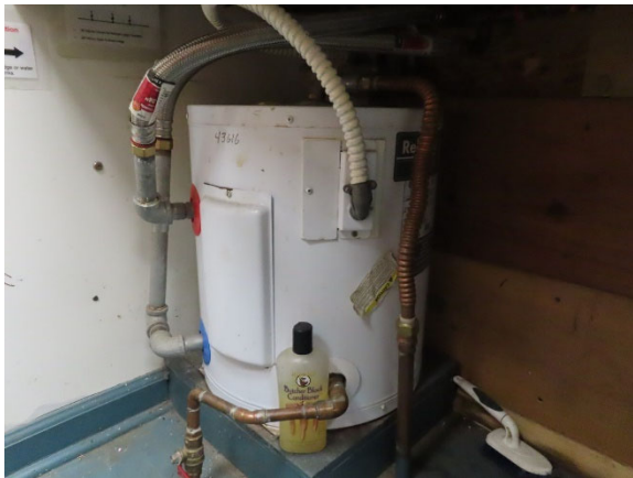
Small 19-Gallon Lower-Level Water Heater
