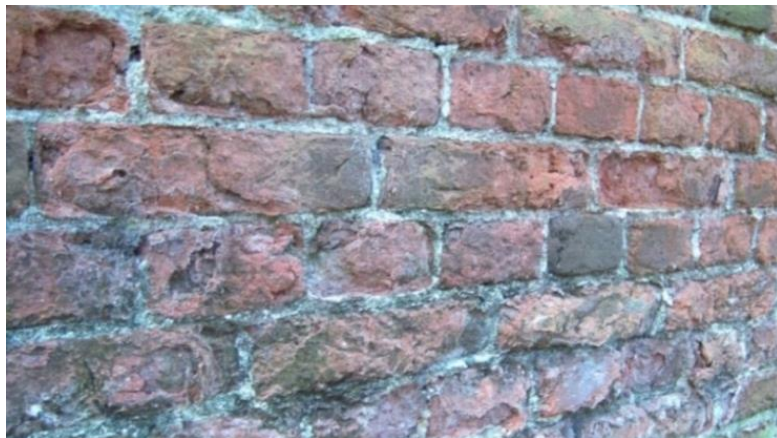
Figure 2.4: Example of frost damage of masonry.
