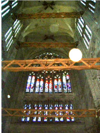
Ad hoc measures preventing the Beauvais cathedral from collapsing.
