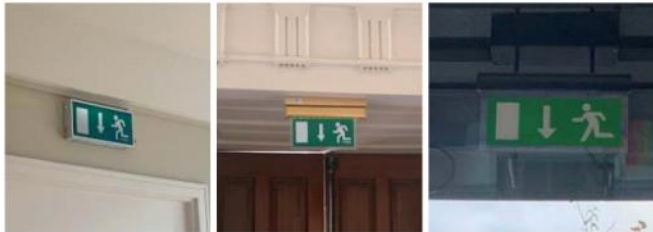
First row of photos shows some emergency exit signs.
