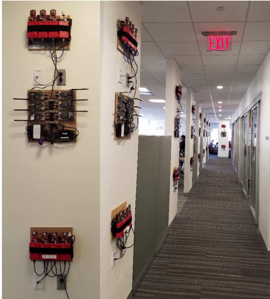
Figure 3.4. Testing Clusters in the Silicon Labs R&D Facility
